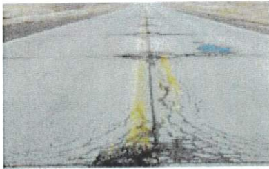
D Cracking - Example 1
