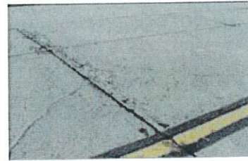
D Cracking - Example 2
